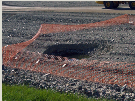
Subsidence found at the base of the embankment
