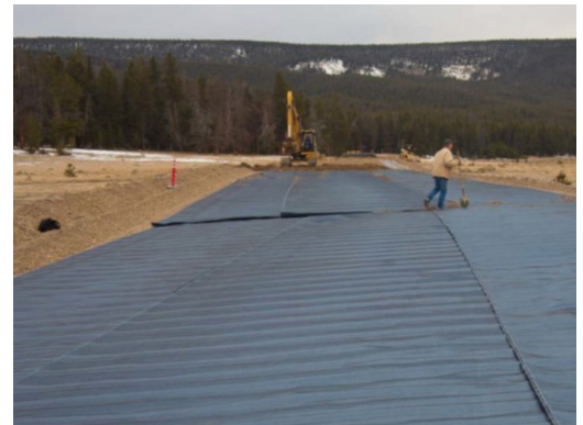
Figure 6(b): Installation of MIRAFI H2Rx with the geotextile unrolled in the direction of the road alignment on the overlapping of geotextile rolls from right to left in a road section with super-elevation on right
