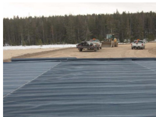
Figure 5(b): Installation of MIRAFI H2Rx with the geotextile unrolled in the direction of the road alignment and middle roll overlapping the two adjacent side rolls in a double cross elevation fall
