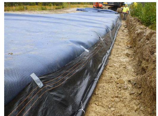
Figure 11(c): Photo of a MIRAFI H2Rx road project with geotextile edge terminated in a saw-cut pipe
