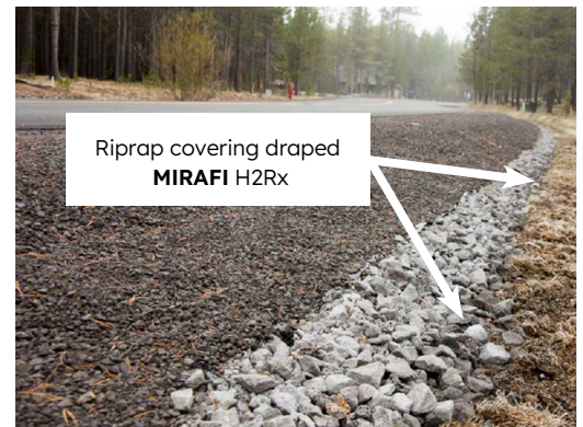
Figure 9(b): Photo of a MIRAFI H2Rx road project with draped geotextile tongue beneath a rock cover
