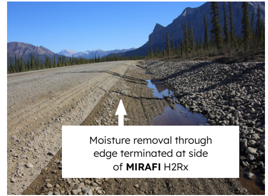
Figure 8(b): Photo of a MIRAFI H2Rx road project with the geotextile edge terminated at side
