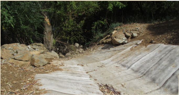
Finished Concrete Canvas installation looking down the drain toward the Lachlan River.
