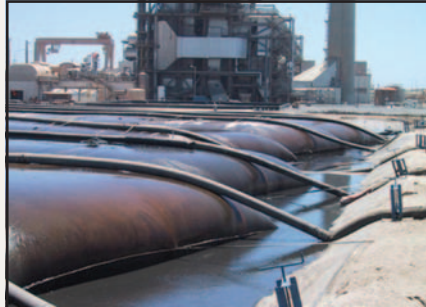
Geotube® containers at fossil fuel power plant being used to dewater fly ash.
